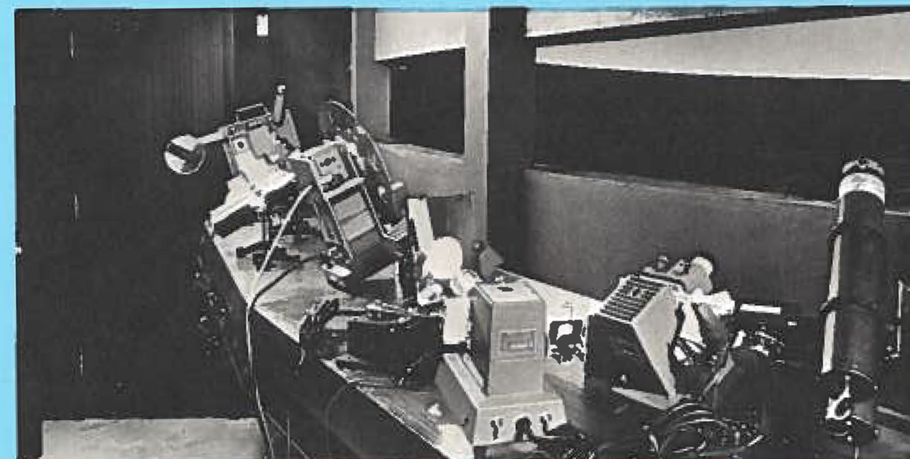
A projection gallery around the theater makes possible the use of dozens of special effects projectors.
