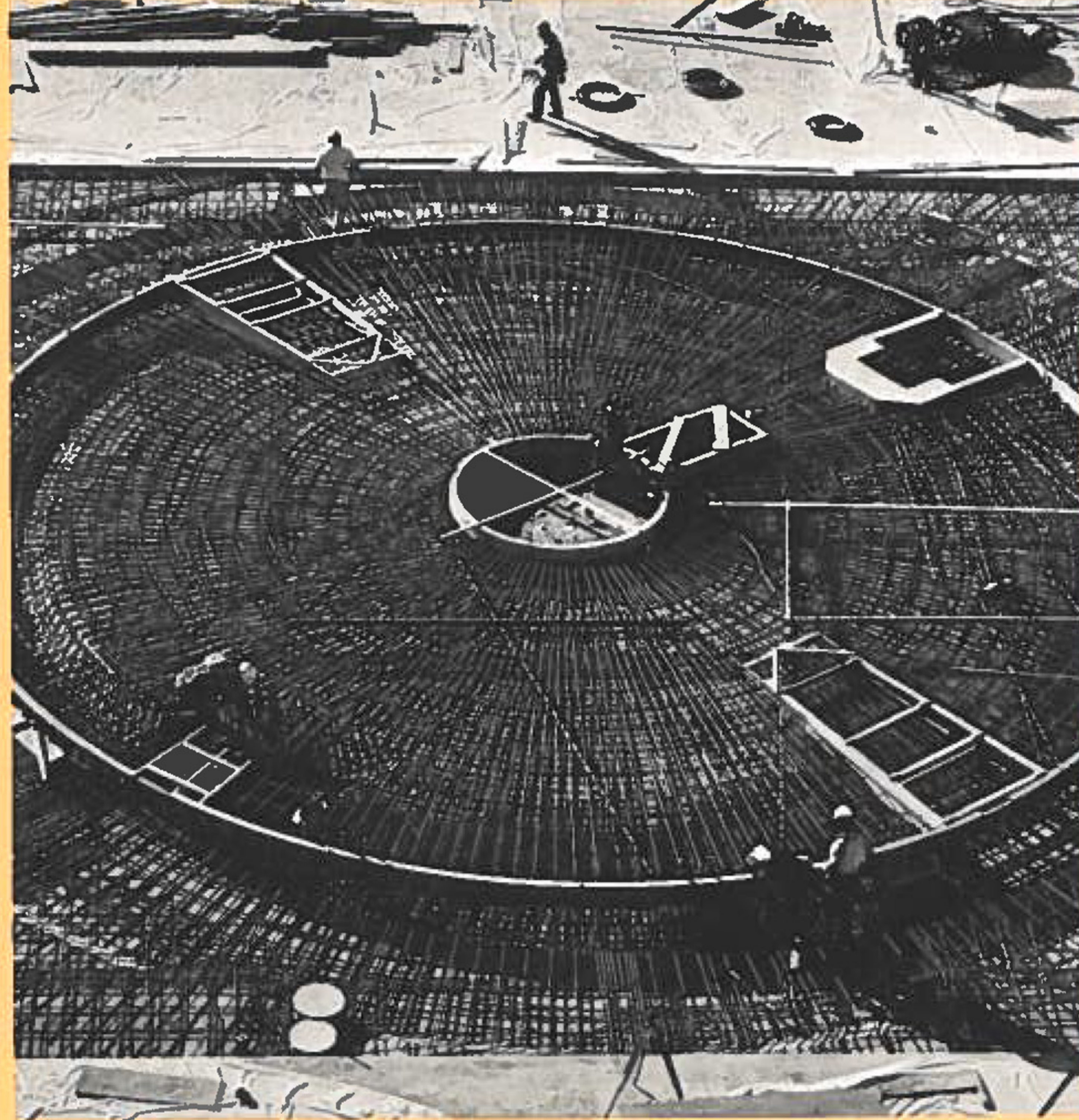
January 1975: Ready for pouring the dome room floor with its radial pattern of reinforcing steel.
